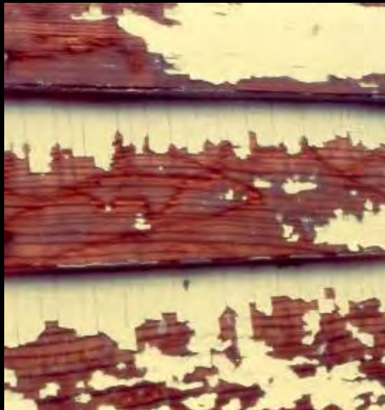
Damage from pressure washer
